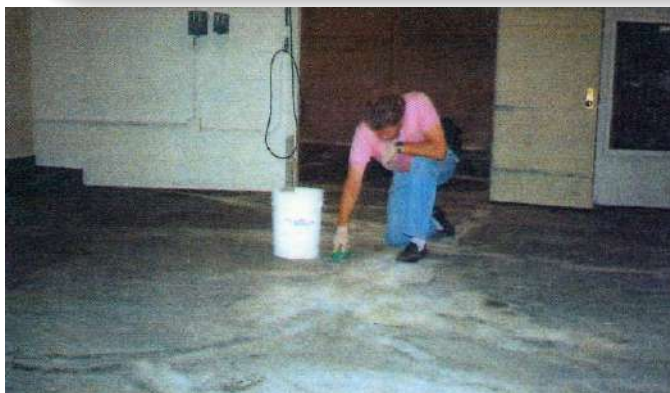
1. An ENECON Field Engineer shows how to make tough floor repairs look easy with DuraQuartz.
