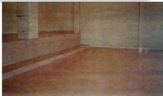
4. The first coat of CHEMCLAD GP (tan color) applied to the entire floor area of the hazardous waste storage
