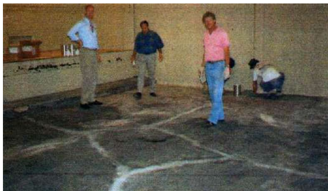
2. A final inspection before the application of CHEMCLAD P4C Primer over the previously repaired concrete floor.
