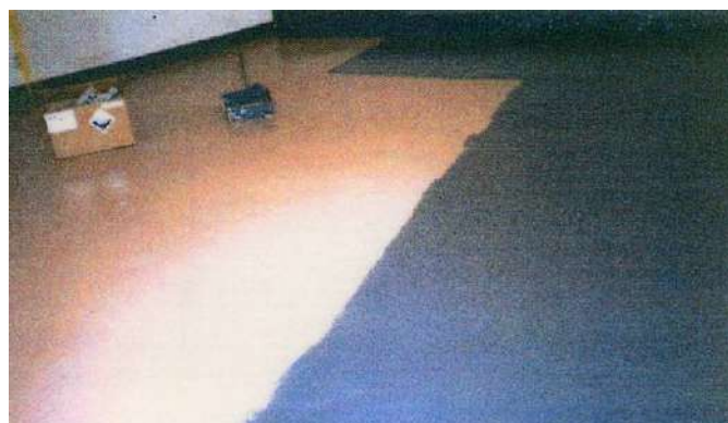
5. The second coat of CHEMCLAD GP (grey color) being applied over the entire floor area.
