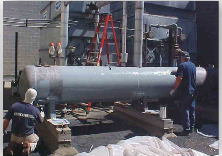
First coat of CHEMCLAD SC being roller-applied to tank and support surfaces.
