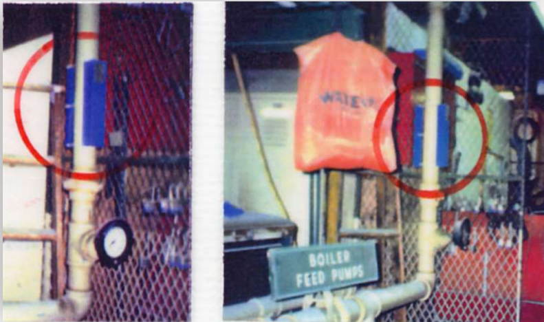
ENEFLOW 5000's installed on boiler feed line.
