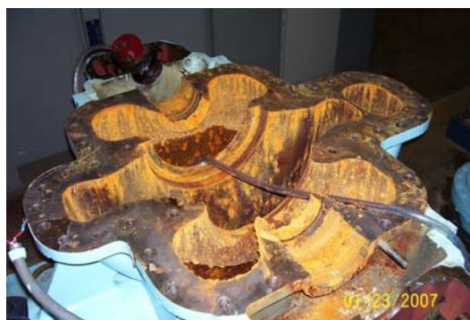
Figure 3-2 Internal Condition of Pump
