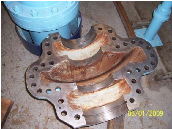
Figure 8-5 Denise Pump Inspection 2009
