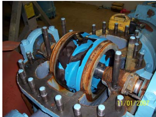
Figure 9-2 Failed Impeller Coating
